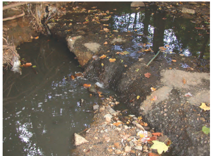
Figure 2. A short-lived sewage source to an unnamed tributary (site S7) to Accotink Creek, Virginia, September 28, 2001.
