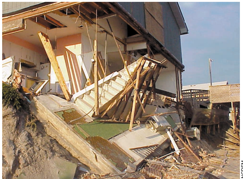
Damaged property at Pine Knoll Shores, N.C., after Hurricane Floyd
