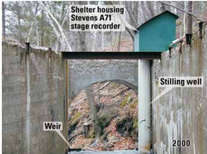
Figure 8. Stilling well and shelter housing instrumentation for gaging streamflow in Nanticoke Creek at Warrior Gap (site 3), Luzerne County, Pennsylvania.
